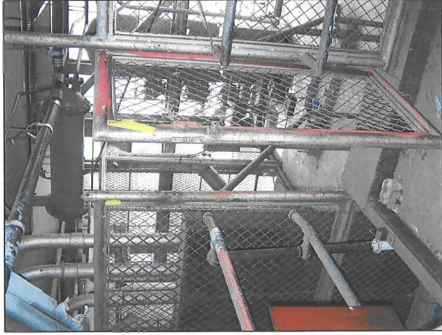
Fence securing mezzanine substations (typ)
