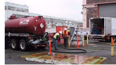
Cleaning and Flushing the G-Line at Pump Station #6, Industrial Wastewater Piping System
