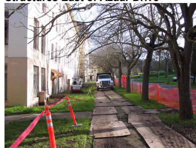
Traffic Controls and Vegetation Protection for Work along Azuar Drive in Touro University Area
