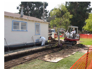
Example of Soil Removal Using Combination of Mechanized Equipment and Hand Excavation around Building P located on Kansas Street
