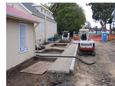
Soil Removal on South Side of Building P located on Kansas Street
