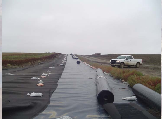
LEADING EDGE OF GEOMEMBRANE, GEOFABRIC AND COVER SOIL ADJACENT TO CURRENT FILL AREA
